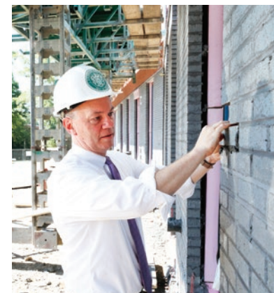
In June, President Conner picked up a trowel to set in place a ceremonial brick in the newly completed east wall.
