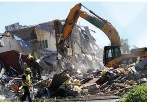
Earlier this year, Skidmore demolished another campus building, Harder Hall, as part of CIS construction.
